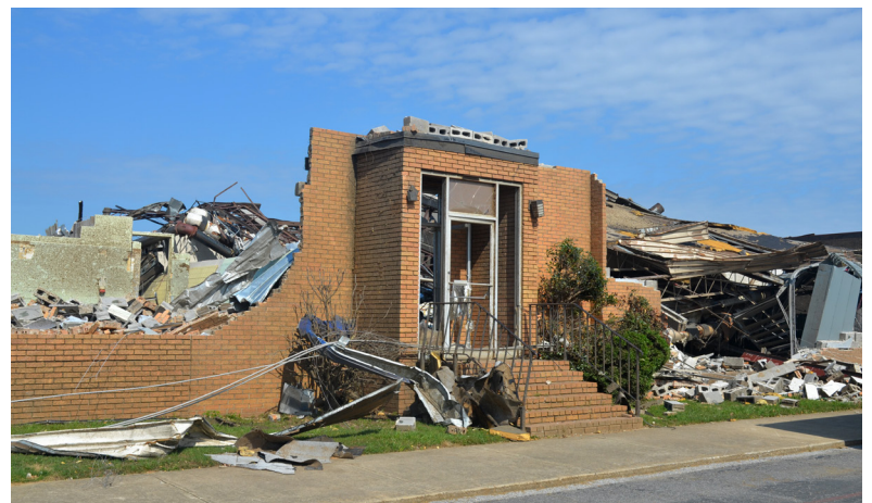
Remains of the entrance to the Curry municipal facility in Tuscaloosa following the April 27th tornado outbreak
